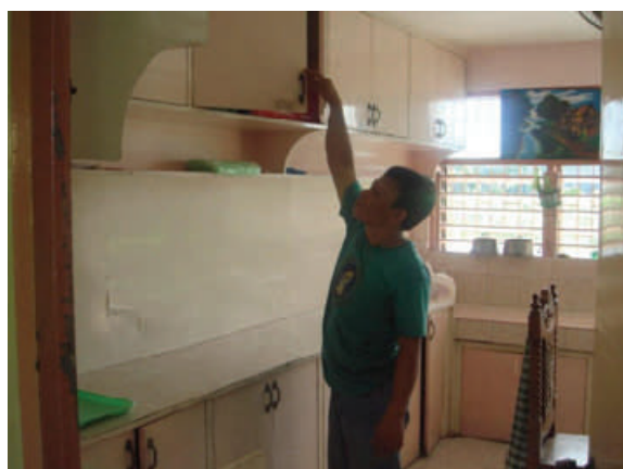
'And the floodwater came up to here'
