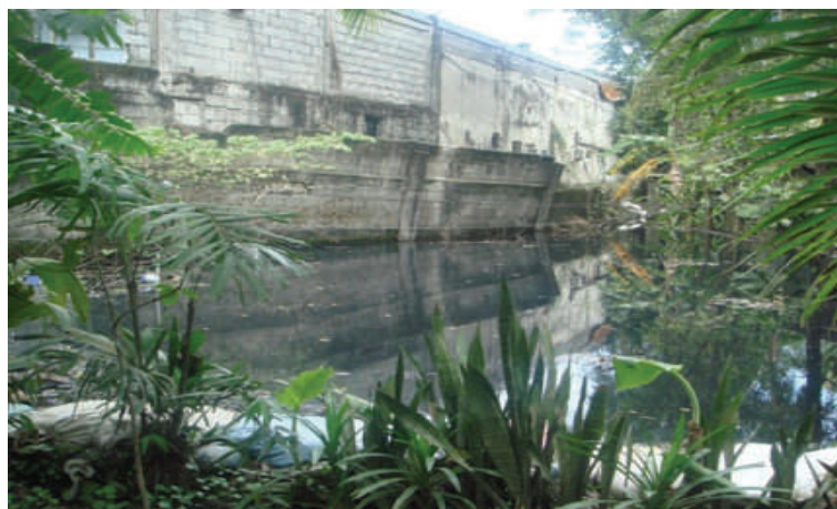
One of the flood defence walls that needs to be urgently replaced
